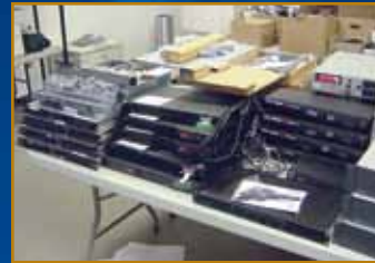
VIEW OF SERVERS & UPS
