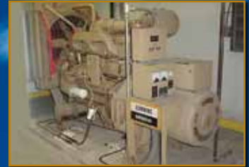
CUMMINS 175 KW GENERATOR SET
