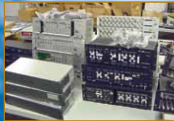
VIEW OF FIBER OPTIC PANELS
