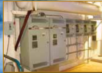
CUTLER HAMMER SV9000 BREAKERS
