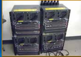
VIEW OF CISCO ROUTERS 4506
