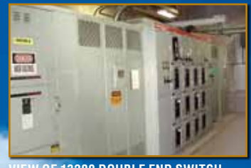
VIEW OF 13200 DOUBLE END SWITCH GEAR SUB STATION
