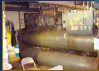
CARRIER 400 TON CHILLER
