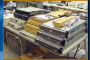
VIEW OF DELL SERVERS
