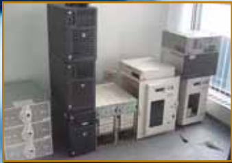
VIEW OF DELL SERVERS
