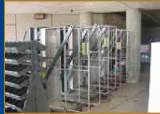
VIEW OF BALLYMORE MAN LIFTS
