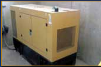
OLYMPIAN D150P1 EMERGENCY GENERATOR
