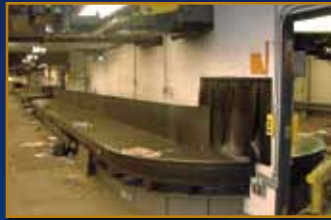
VIEW OF BAGGAGING HANDLING CONVEYORING
