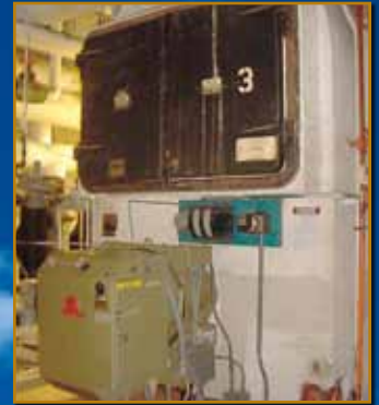
VIEW OF PACIFIC NATIONAL STEEL BOILER
