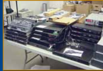
VIEW OF SERVERS & UPS
