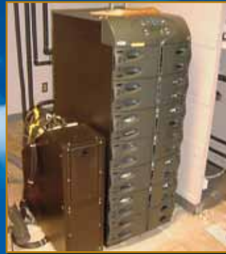
INFINITY EMERG. POWER BACKUP SYSTEM
